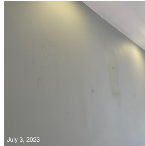
PAINTED OVER DEFECTS
