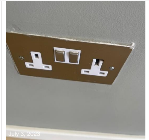
CRACK TO SOCKET (RHS)
