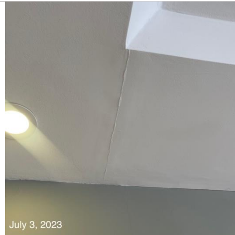
CRACK TO CEILING
